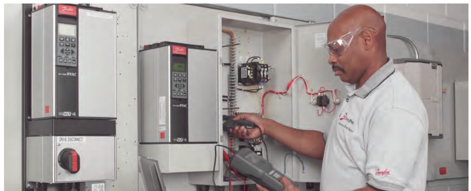
The DrivePro™ Service organization is committed to ensuring complete customer satisfaction
