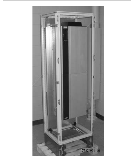
3.36: Adjustable frequency drive installed in cabinet
