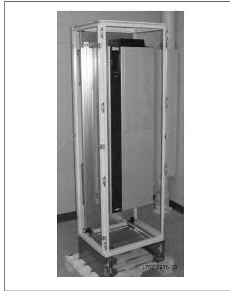
3.36: Adjustable frequency drive installed in cabinet
